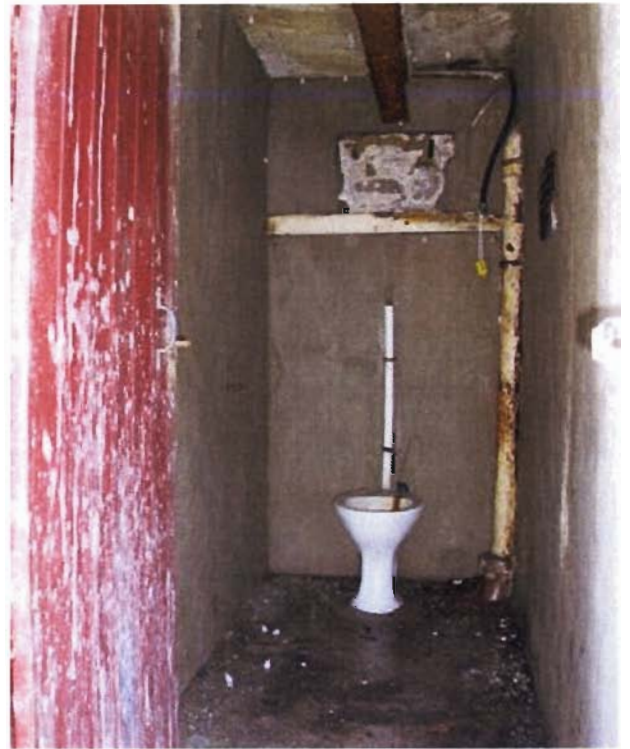
Toilet to right side to be retained, repaired and re-plastered, with fittings.
