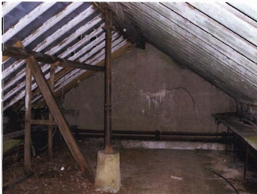
First floor space looking to west gable. Rafters to earlier glazed roof to be retained below new roof structure to take slate roof. Exg. ridge beam retained and strengthened. Render finish to walls to be removed to take insulated lining.
