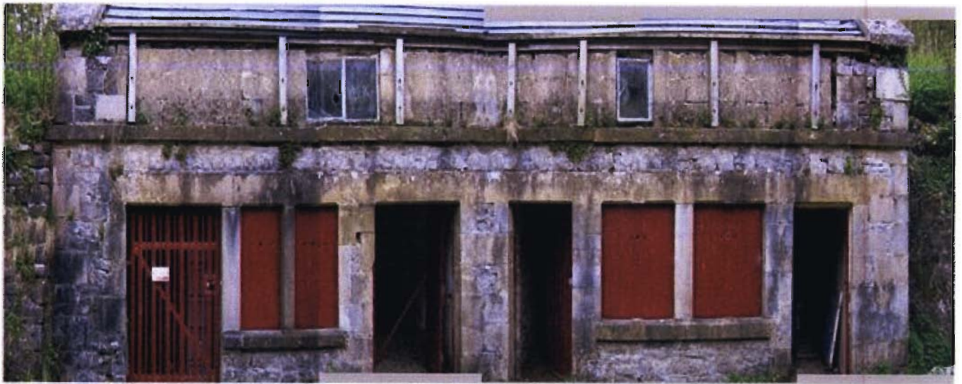
Main elevation showing missing mullions to right hand window openings at ground floor. Boarding to openings to be replaced to left hand side by new painted glazed timber casement windows as exg. consent and new stained glass panels in softwood frames to right hand side . Blockwork infill to first floor to be replaced by new painted double glazed fanlights.
