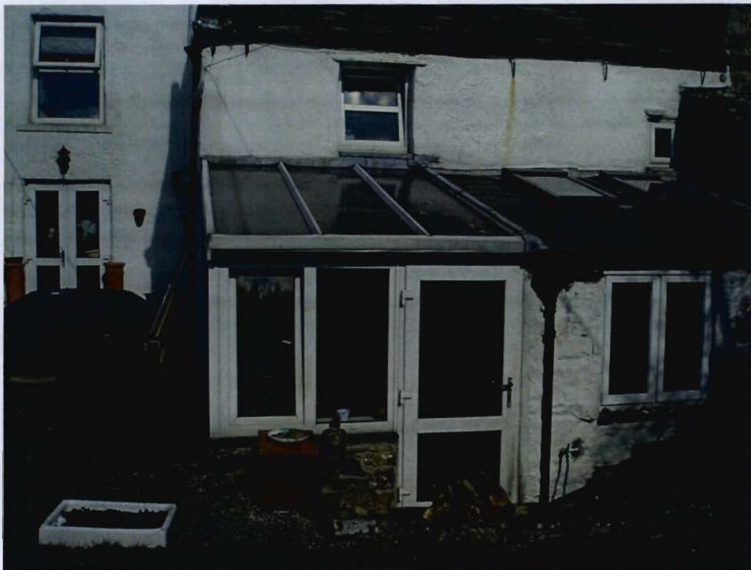
Rear view showing existing upvc conservatory and location of new dining area
